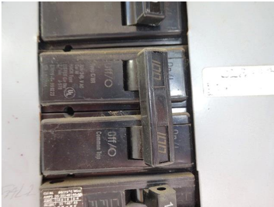
Electrical: Main breaker 100 amp
