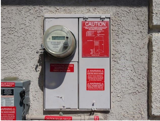
Electrical: Main Panel
