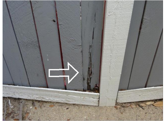
Fences / Gates: Area of wood rot to fence slat.
